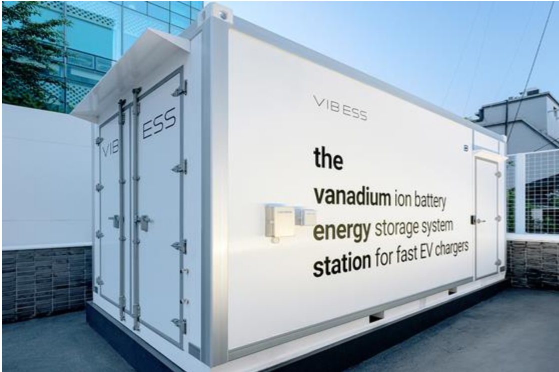
An energy storage system powered by vanadium-ion batteries installed at Lotte Himart in Apgujeong, southern Seoul [STANDARD ENERGY]
